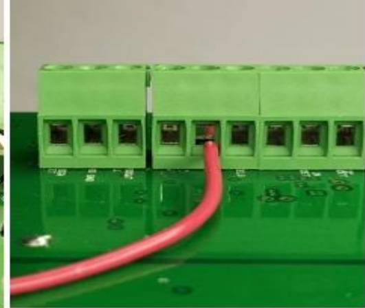
BAD, WIRE "UNDER" SCREW CLAMP
