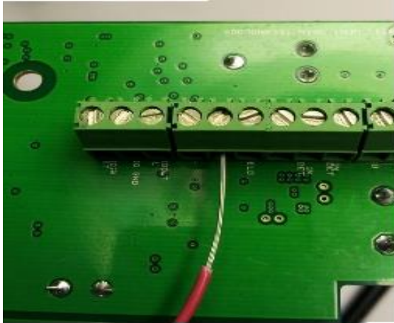
BAD, WIRE STRIPPED TOO FAR
